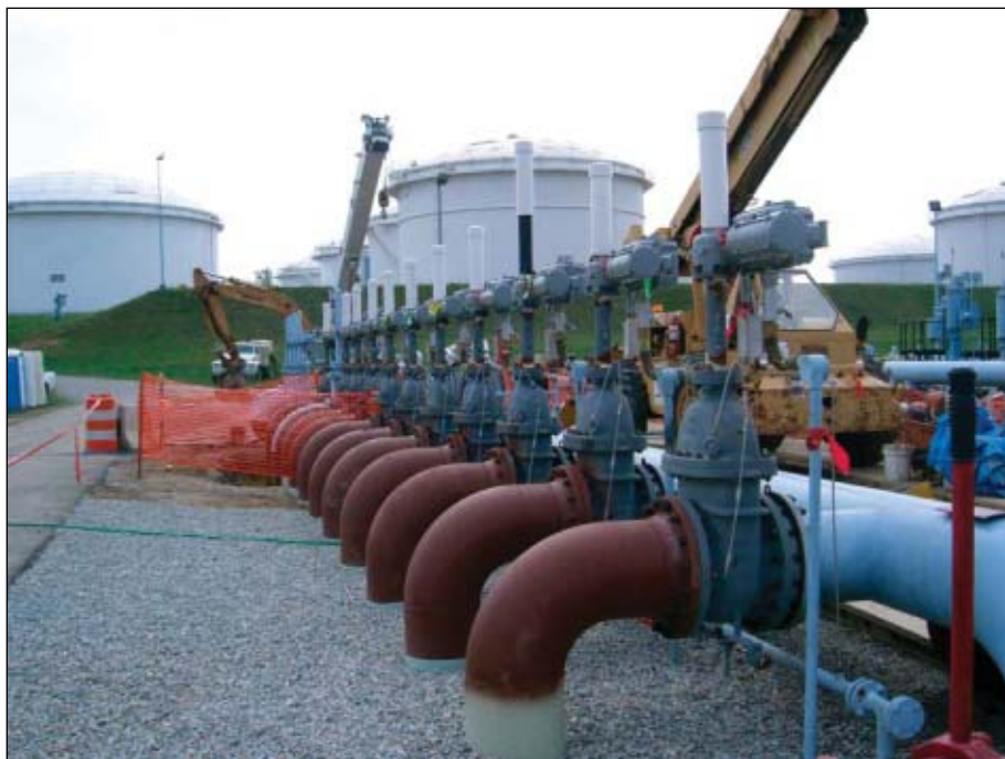
Colonial Pipeline Co. replaced more than 300 valves in preparing to transport ultralow-sulfur diesel. The new valves are positive-sealing valves, which minimize any contamination of ULSD by other products. This picture shows Colonial's out-going valves on Line 27 at Mitchell Junction in central Virginia (Fig. 4; photo from Colonial Pipeline Co.).
