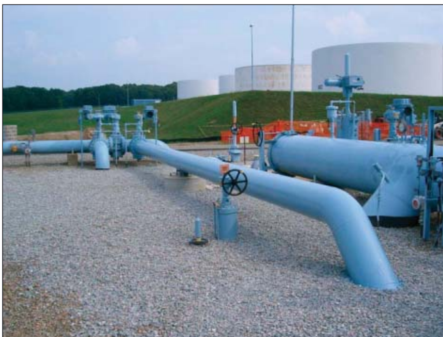
Transportation of ULSD via pipeline heightens any potential product-quality problems on the pipeline's systems, making proper flushing of prover loops such as the one shown here very important (Fig. 6; photo from Colonial Pipeline Co.).
