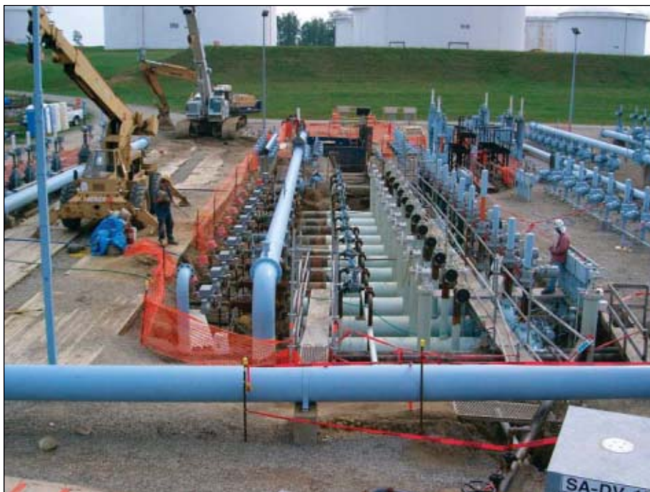
Proper change-of-service procedures for ULSD required a detailed design review of each pipeline manifold, such as that pictured at Colonial's Mitchell Junction in central Virginia. In addition to using positive-sealing valves, the elimination of dead legs helps ensure effective manifold flushing (Fig. 5; photo from Colonial Pipeline Co.).
