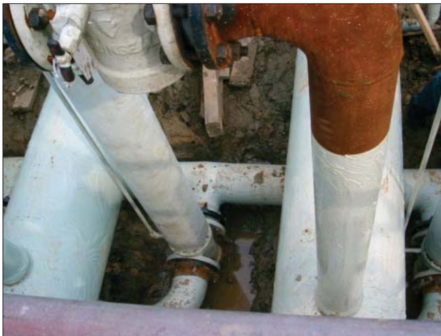
Colonial Pipeline Co.'s preparations to transport ULSD included installation of new transfer system components, including the 10-in. line shown (Fig. 7; photo from Colonial Pipeline Co.).
